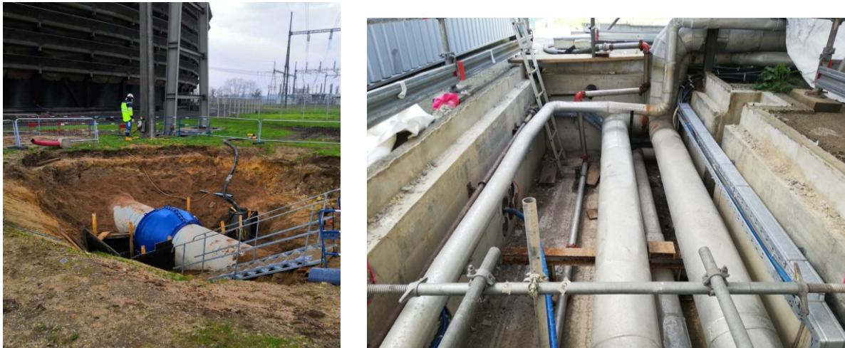
Figure 1-4: Service water pipes, buried or in galleries.
