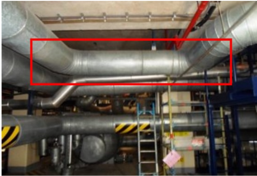
Figure 3-3: Images of the high-pressure steam turbine extraction line.
