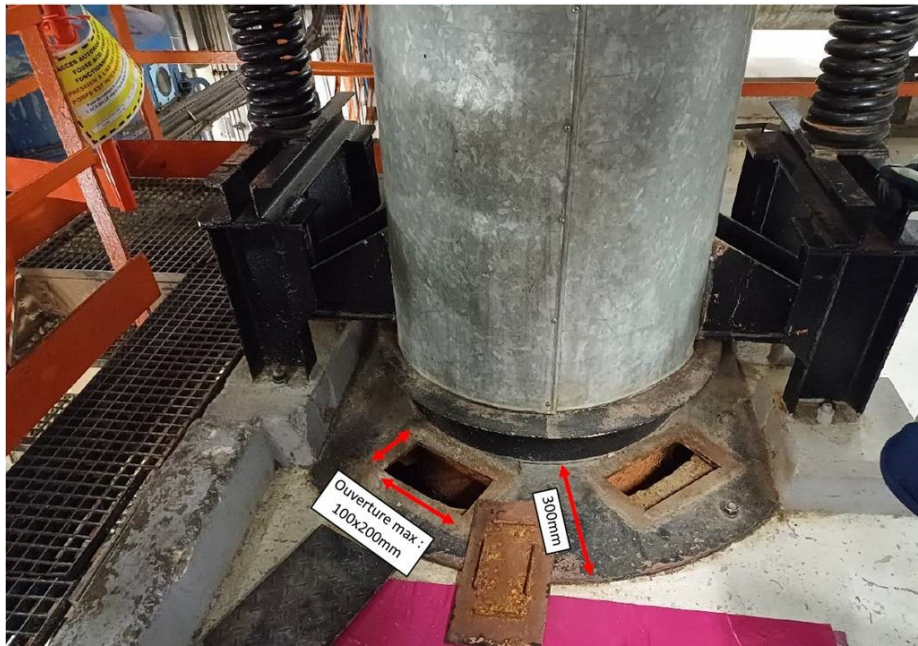
Figure 2-1: Preheater siphon in place with heat insulation.
